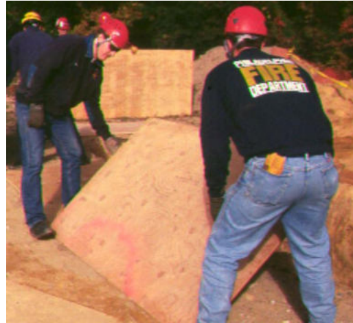
Marking ground pad
