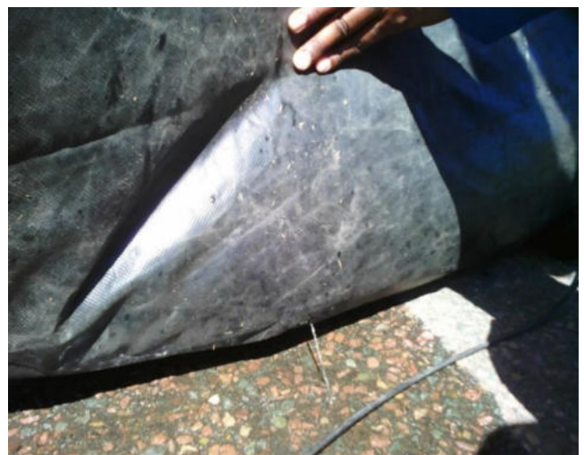
Leak in the Fast Tank
