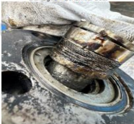
Damaged Mechanical Seal
