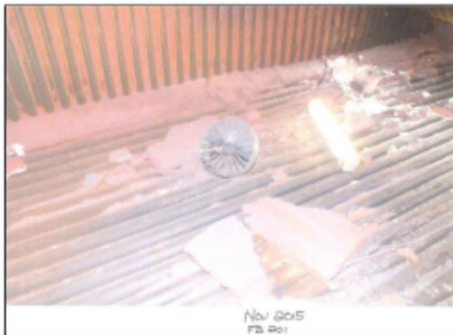
Photo 13: - "Missing" Air Swirler lying on Boiler Floor
