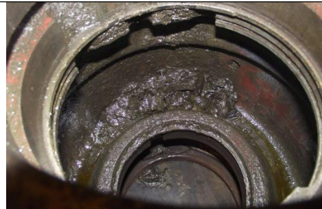
Sludge inside bearing housing
