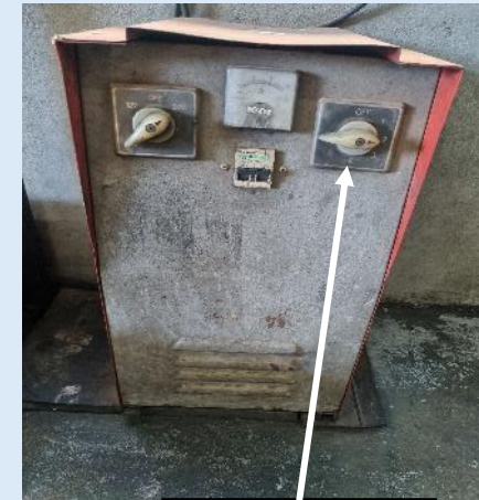
Battery charger was set at 24 volts to charge two batteries
