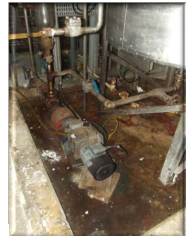
Faulty Pump per MOCA
