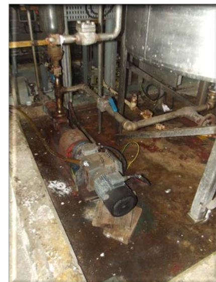
Faulty Pump per MOCA
