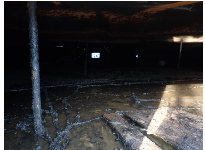
2: Slippery substance on the tank floor
