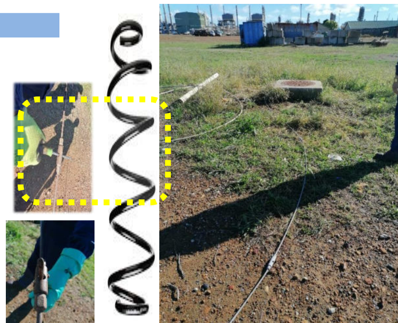
Rod length outside manhole: Length too long outside manhole.
