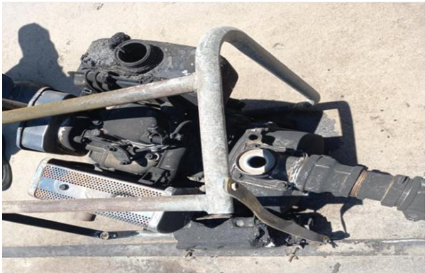
Picture 2: Burnt Generator used during meter
