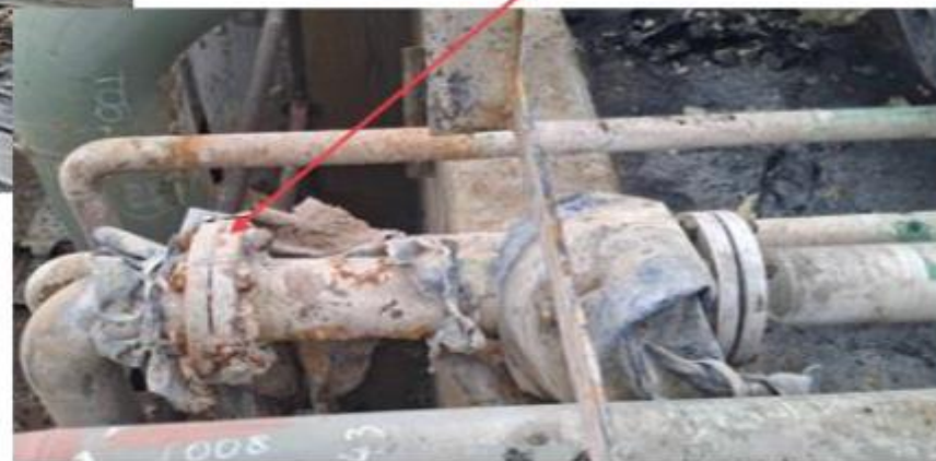
Sulphuric acid leaked flange
