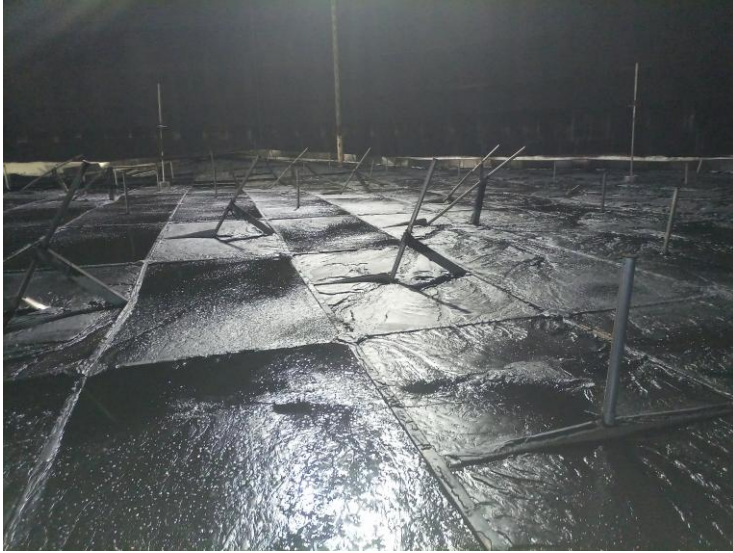
IFR roof legs
