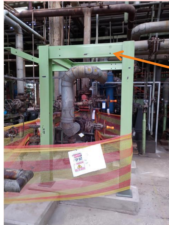
Crossbeam which detached and fell
