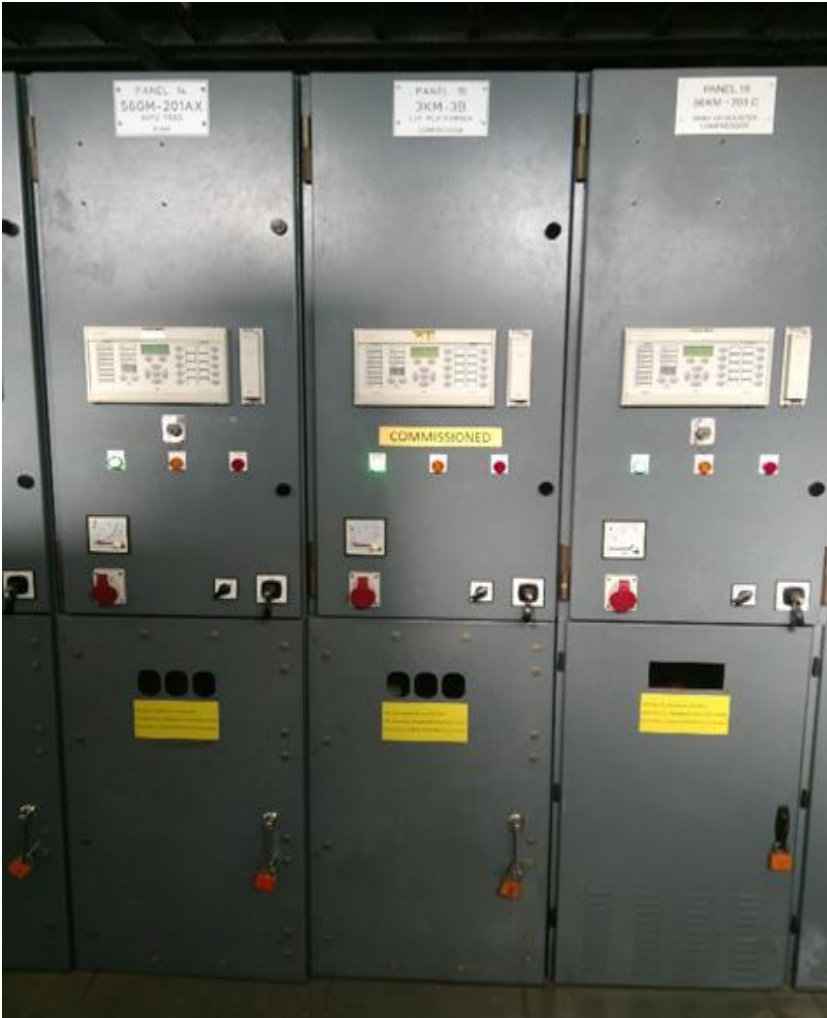
3KM-3B panel in the substation
