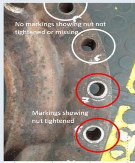
Lack of markings showing nut not tightened or missing
