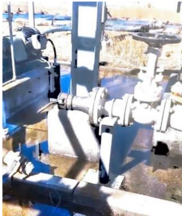
Flexible hose connection point slightly outside the bunded area
