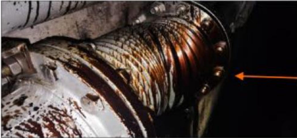
Bellows in the 10 inch VLSFO line
