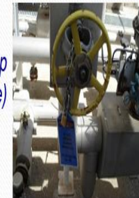
Operation group lock & tag (blue) at the valve
